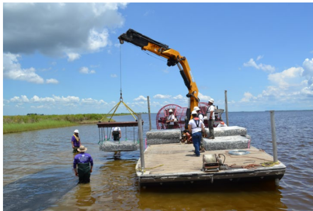
Figure 3. As part of oyster reef restoration efforts in Calcasieu Lake, Louisiana, a construction and engineering crew placed gabions – wire cages filled with rocks – in the intertidal zone to construct substrate for growth of larval oysters. Photo courtesy of The Nature Conservancy.
